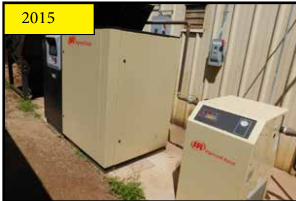
2015 IR R45I-A125, 60 HP ROTARY AIR COMPRESSOR WITH DRYER.
